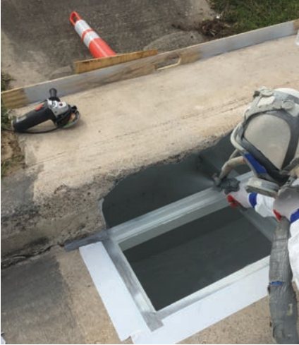
Fig. 3 (above): In addition to the pipe interiors, the contractors also spray-applied coatings to catch basins, manholes and other related structures.
